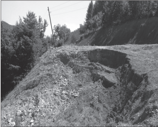
Figure 1: Slope sliding after reconstruction of the road section Krupanj-Ljubovija (source: author)
